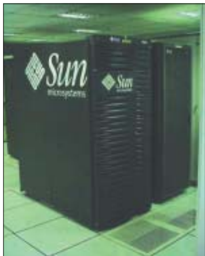
Sun servers at the TTSL facility
